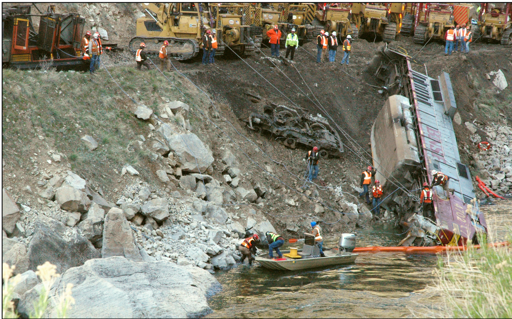
Seven cranes were used to lift railroad cars back onto the tracks after the derailment of a Burlington Northern-Santa Fe train last week. There were no injuries in the accident
